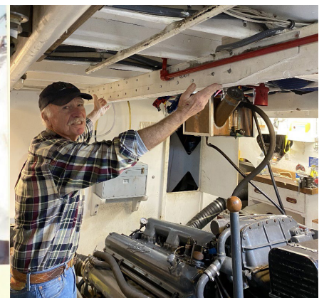
Crewmember Steve Stange pointing out the repaired stringer in the engine room
