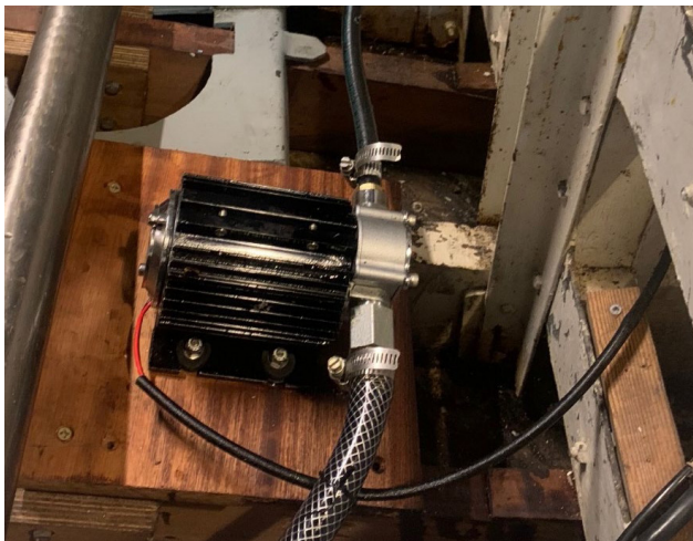
Pre-lube pump installed close to the lube oil sump and engine.
